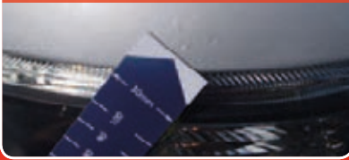
Poor repair: paint blisters around lamp
